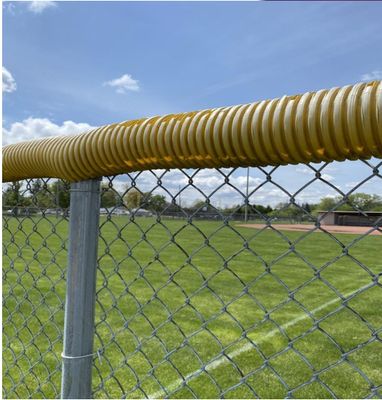
Eroded fence capping
